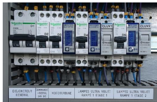
Figure 3: circuit breakers in the electrical compartment
